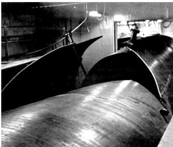
Fig.10. Welded joint failure
