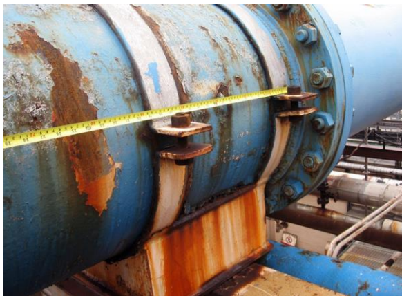
Fig.11. Failure due to corrosion and cracking
