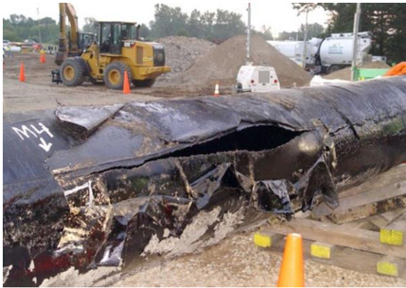
Fig.12. Failure due to use of poor quality of materials
