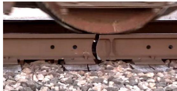
Fig 2: Railway Track Crack
