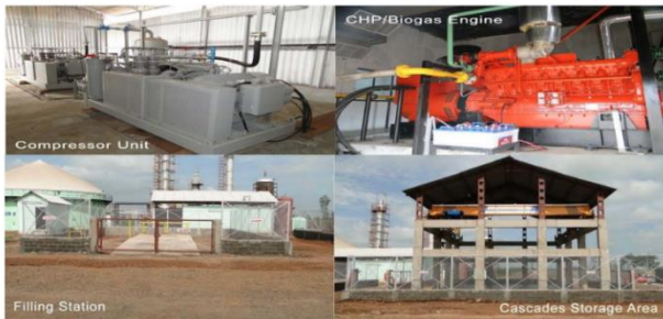
Fig. 3. Inside Bio Cng Plant
