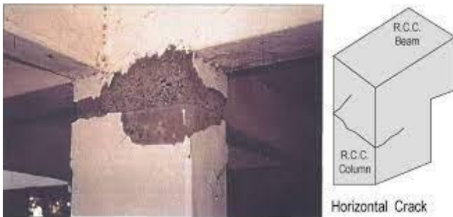
Figure-2 Crack of Column
